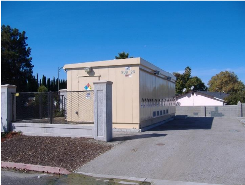
Figure 7-27. Visual Elements: Typical Substation
